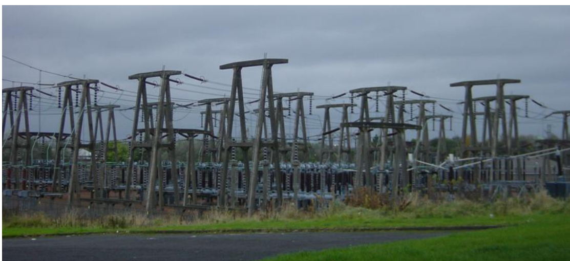
The Substation adjacent to Allershaw Road
