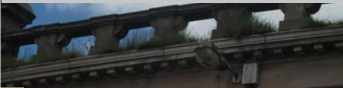
5 Vegetation damaging stonework.
