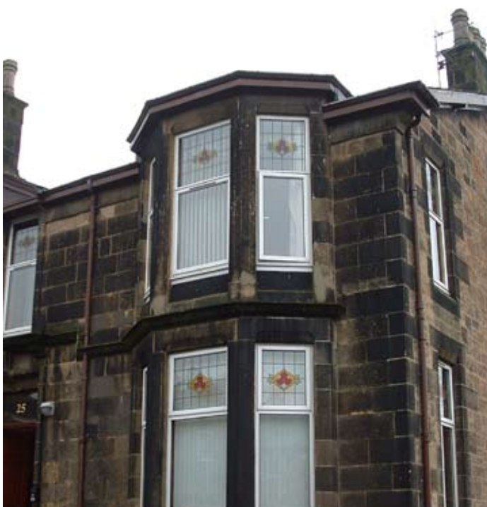
In some instances windows are replaced with UPVC without consent, which would be a breach of regulations and may cause difficulties with a future sale.
