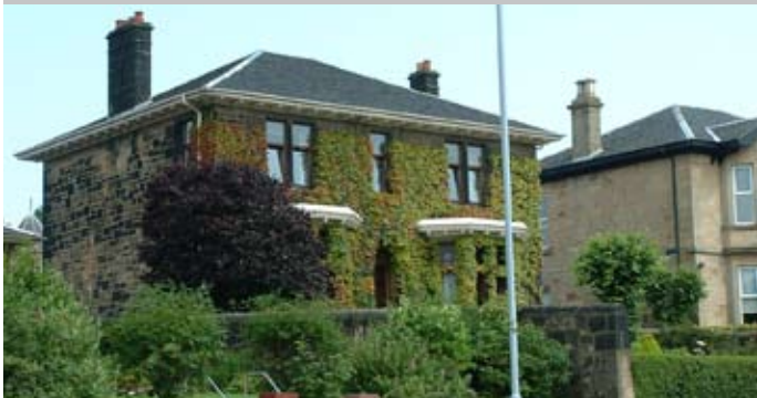
Ivy can penetrate and damage stonework.
